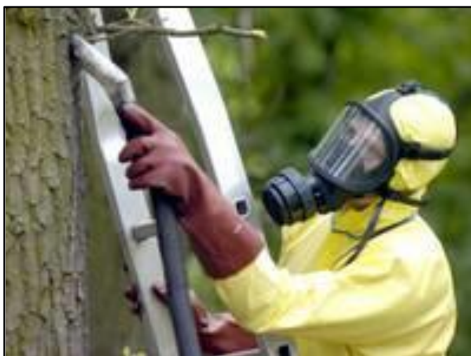
Vacuum removal of OPC uses special equipment and full personal protective gear
